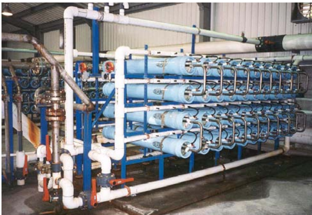
Figure 1: The Zeta Rod™ protects a wide range of Reverse Osmosis units, including this system used for drinking water production in the Caribbean.
